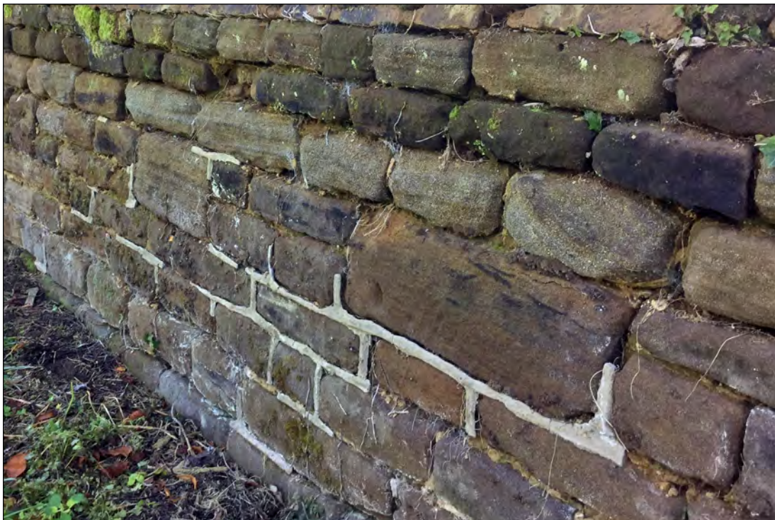
C.05: OPEN JOINTS & FAILING CEMENT MORTAR IN NEED OF RENEWAL
