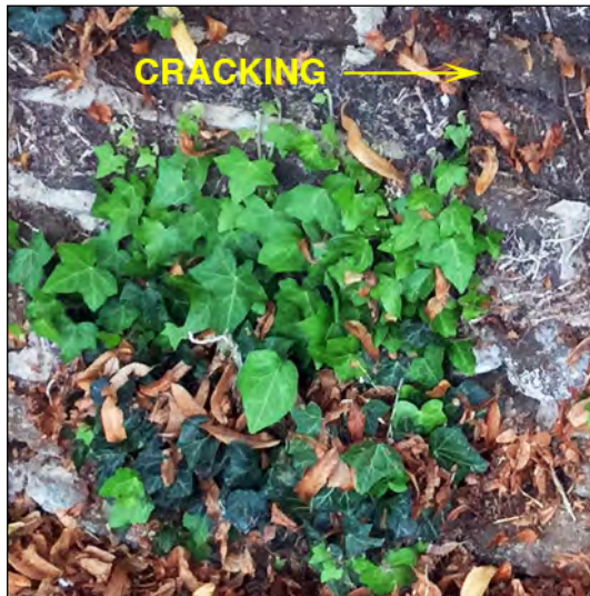
C.01: IVY PENETRATING JOINTS
