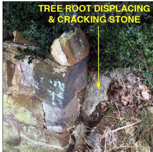
C.02: HOLLY TREE DAMAGING WALL
